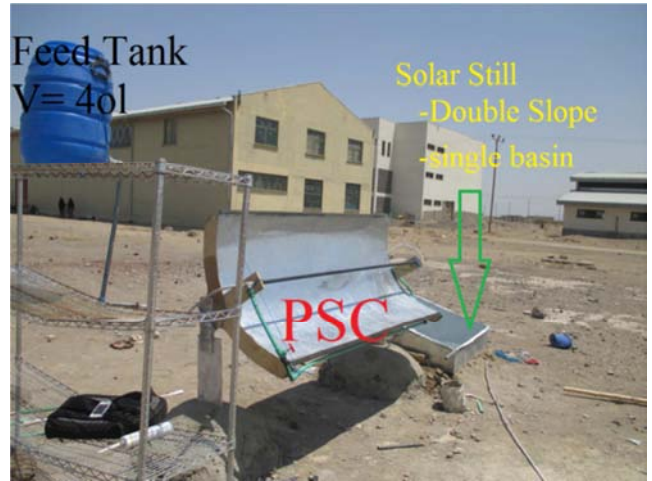
Figure 4. Installed Active Solar Still.
